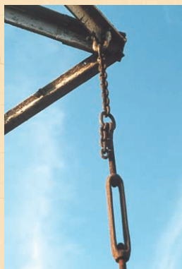
Remnant of the corner hold-down chain
